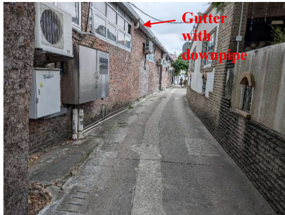
Plate 5 – Existing 225mm channel running along the eastern boundary of the Application Site flowing to the north. Existing gutter at the roof edge of the ‘Red Brick House’ with downpipes discharge into the existing channel.
